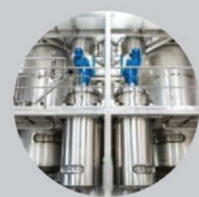
Biorefinery Pilot Plant
